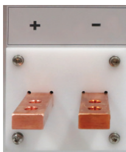
DC tin plated copper bus bars installed in back panel
